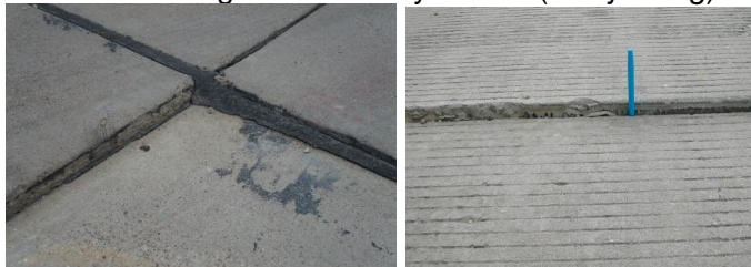
Gambar III.32 Penurunan Slab di Sambungan ( Stepping at Transverse Joints )
