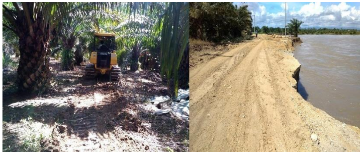
Gambar III.27 Gerusan ( Erosion Gullies )
