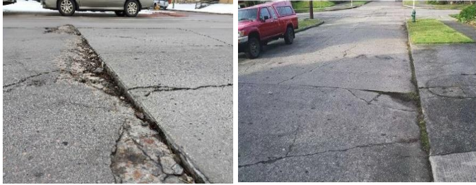
Gambar III.33 Slab Pecah dan retak di sambungan ( Spalling at Joints and Crack )
