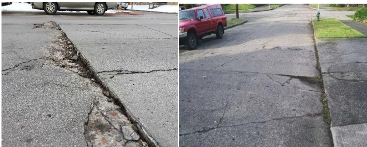
Gambar 3. 33 Slab Pecah dan retak di sambungan ( Spalling at Joints and Crack )
