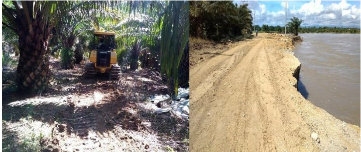
Gambar 3. 27 Gerusan (Erosion Gullies)
