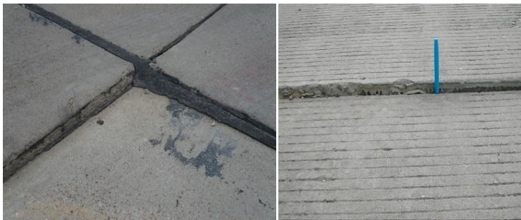
Gambar 3. 32 Penurunan Slab di Sambungan (Stepping at Transverse Joints)
